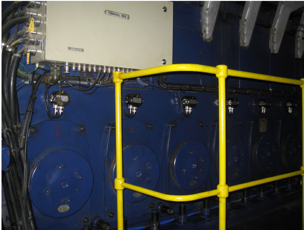
Fig. 5.12 Installed Sensor of SiCOMS® System on a 4 stroke engine
