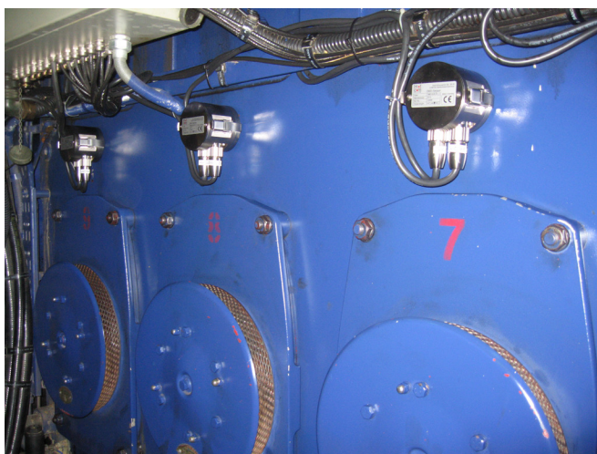
Fig. 5.1 Example of Installation for Sensors and SOG
